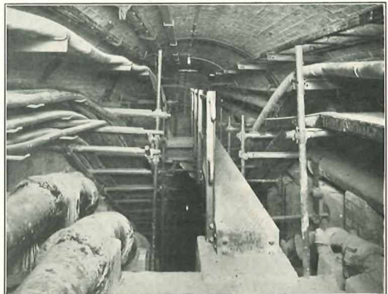
FIG. 18.—STREET APPROACH SHOWING TUBULAR CABLE SUPPORTS.
