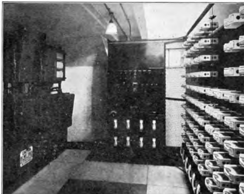
FIG. 9.—BASEMENT SWITCHROOM—GENERAL RESEARCH BUILDING, SHOWING "SPECIAL VOLTAGE" PANEL IN CENTRE, PART OF A.C. SWITCHROOM ON LEFT, AND D.C. DISTRIBUTION PANELS ON RIGHT.
