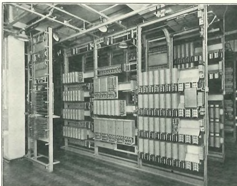
FIG. 3.—TYPICAL EQUIPMENT AT A KEYSENDING CENTRE.
