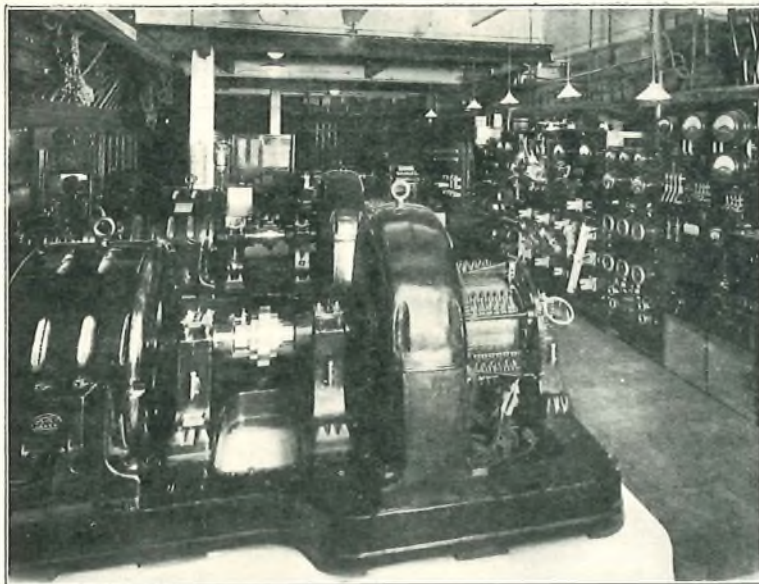
FIG. 3.—GENERAL VIEW OF POWER PLANT.
