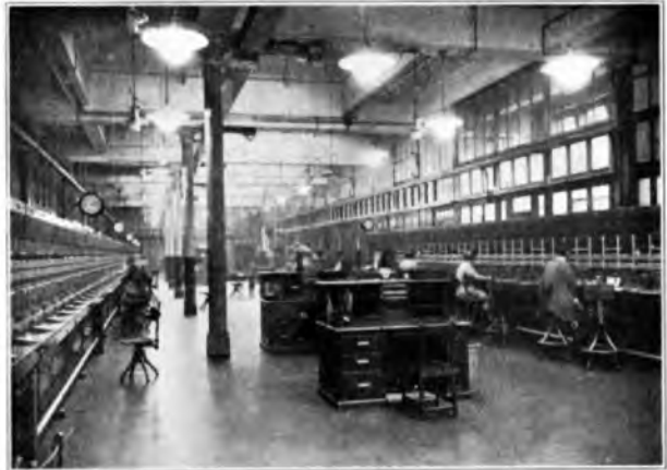
FIG. 4.—TELEPHONE TRUNK SWITCHROOM.
