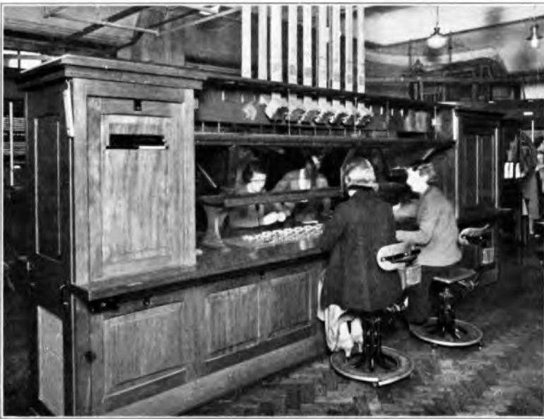
FIG. 4.—P.D.P. IN INLAND TRUNK EXCHANGE CONVERTED FROM MIX AND GENEST TO MCGREGOR TERMINALS.
