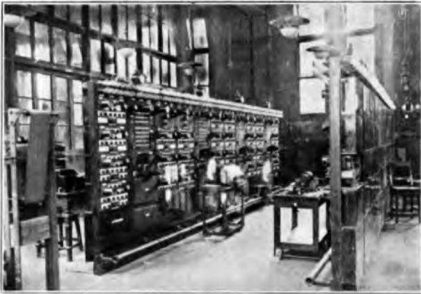
FIG. 2.—TELEGRAPH ROOM; RACK-MOUNTED APPARATUS.
