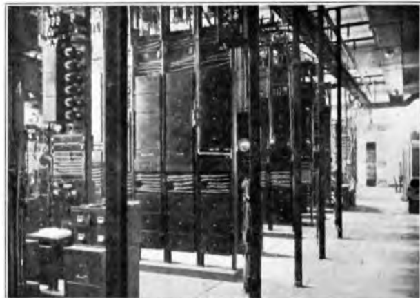
FIG. 6.—REPEATER ROOM, INCLUDING V.F. TELEGRAPH AND TARIFF "A" PRIVATE WIRE RACKS.
