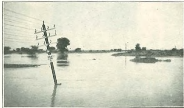
FIG. 12.—LINES DAMAGED BY FLOODS.
