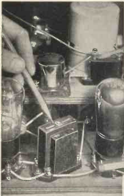
Here you see the compensating L.F. transformer which is an integral part of the tone-leveiling system which plays an important part in making the K4 the outstanding design of the year.
