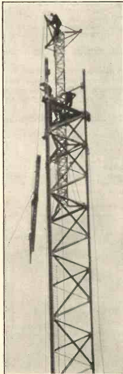
One of the masts in the course of erection on the site of the B.B.C.'s new high-power long-wave station at Wychbold They are to be 700 ft. high!
