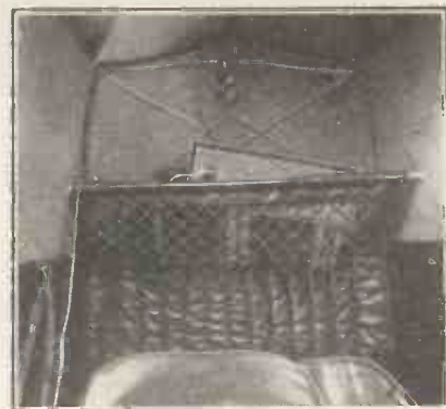
The battery box is easily accommodated on the luggage rack, in the locker, behind a seat, or anywhere convenient. The plug makes it quickly removable, if necessary, without upsetting the armoured cabling.
