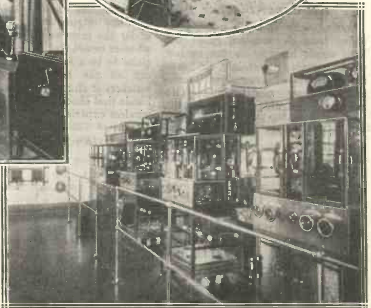
To the right is a view of the main transmitter, which is of British manufacture, and greatly resembles some of the older B.B.C. transmitting plants. But except from an engineering point of view, Bombay's broadcasting problems are entirely different from ours, including as they do the difficulties of languages and of castes.
