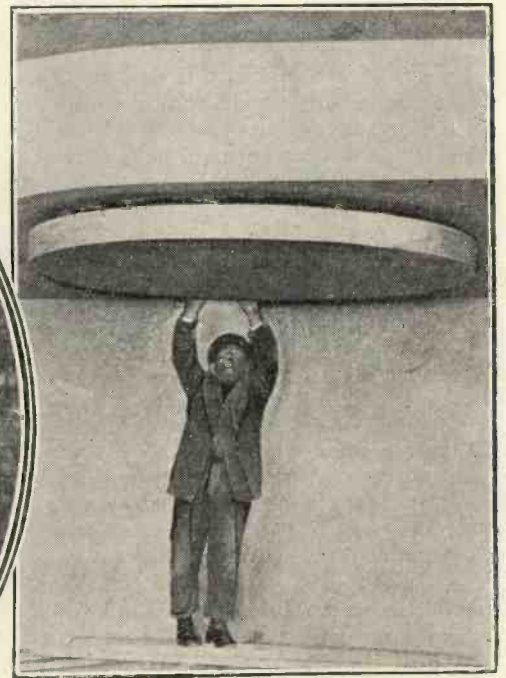
(Top) The B.B.C.'s new Broadcasting House is nearing completion, as you will see from this recent photograph. (Bottom, left) Part of the ingenious and complicated ventilating system. (Bottom, right) The end of a ventilation duct in a studio ceiling.
