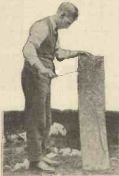
Earthing plates should be buried in soil which is always damp, otherwise the efficiency of the earth will vary greatly.
