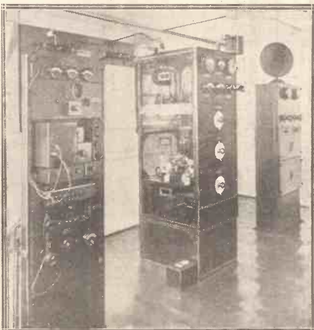
The neatness in wiring, etc., remarked upon by our special representative is well illustrated in this view of Auckland's transmitting gear.
