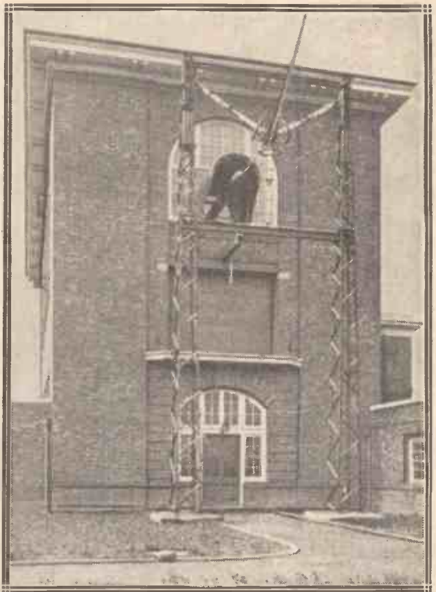
The aerial "lead-out" at the Rugby station. Note the huge insulators supported on a framework resembling miniature masts.
