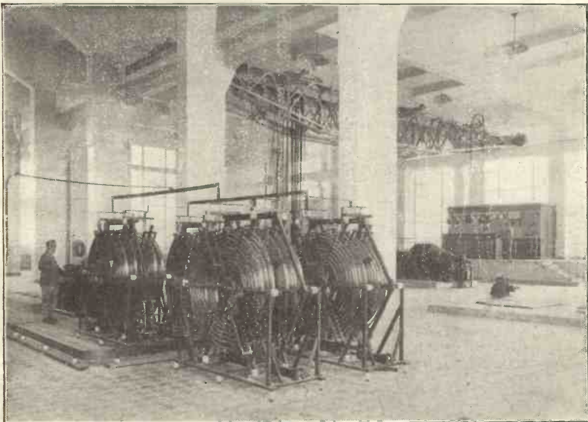
The giant aerial tuning inductances at the St. Assise station, near Paris. This station communicates direct with America.
