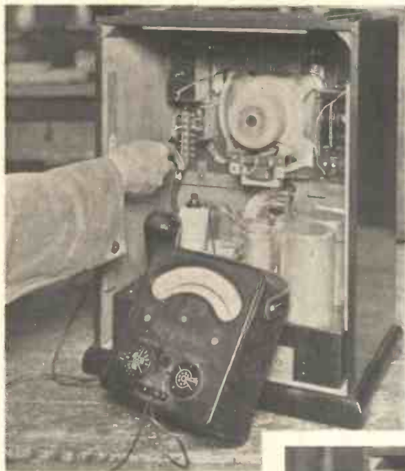
Fig. 6.—TESTING VOLTAGES AT THE TERMINAL STRIP.
