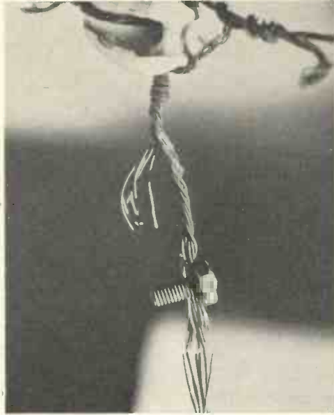
Fig. 9.—A FAULTY DOWN-LEAD THAT MAY GIVE TROUBLE.
