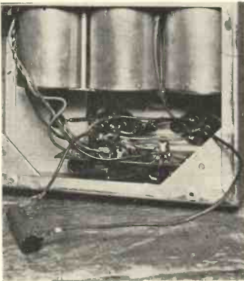
Fig. 20.—TESTING 0.1 CONDENSERS ON H.F. PANEL.
