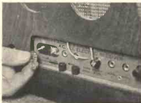
Fig. 3. —THIS SHOWS THE POSITION OF THE MAINS FUSE WHICH IS FITTED ON THE TERMINAL STRIP BEHIND THE SET.
