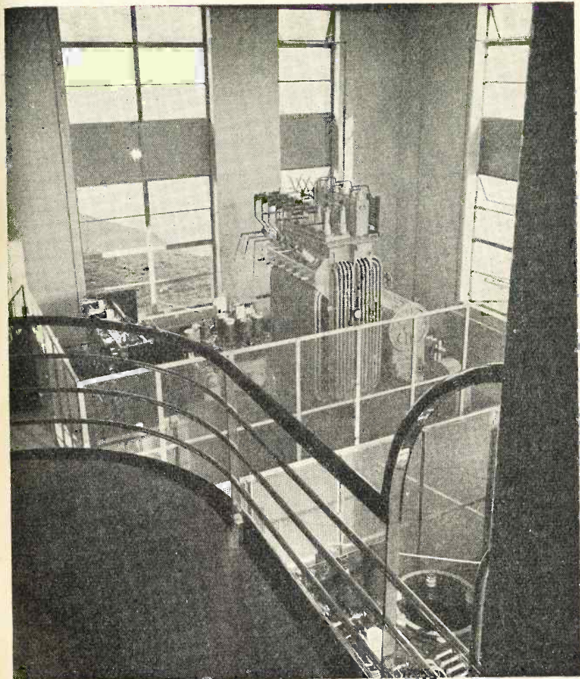
A dramatic view of part of a transmitting station. The large piece of equipment near the corner of the hall is a transformer for one of the mercury-arc rectifiers which provide a high-tension supply at 20,000 volts.
