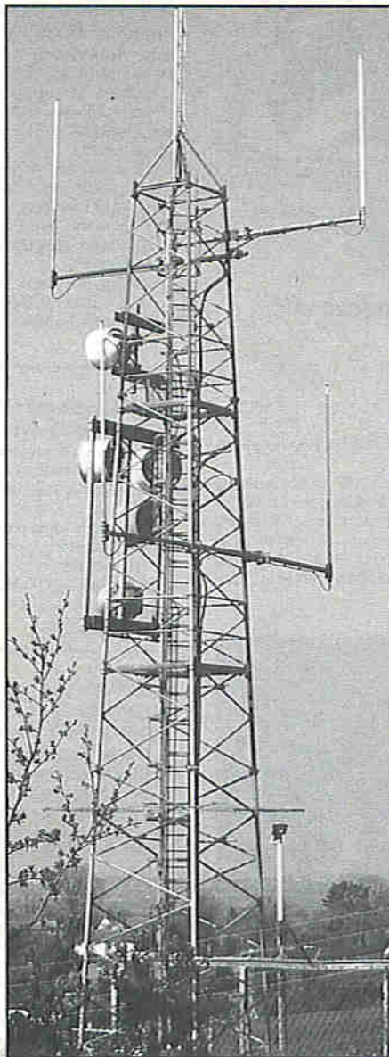
Typical base station site.
