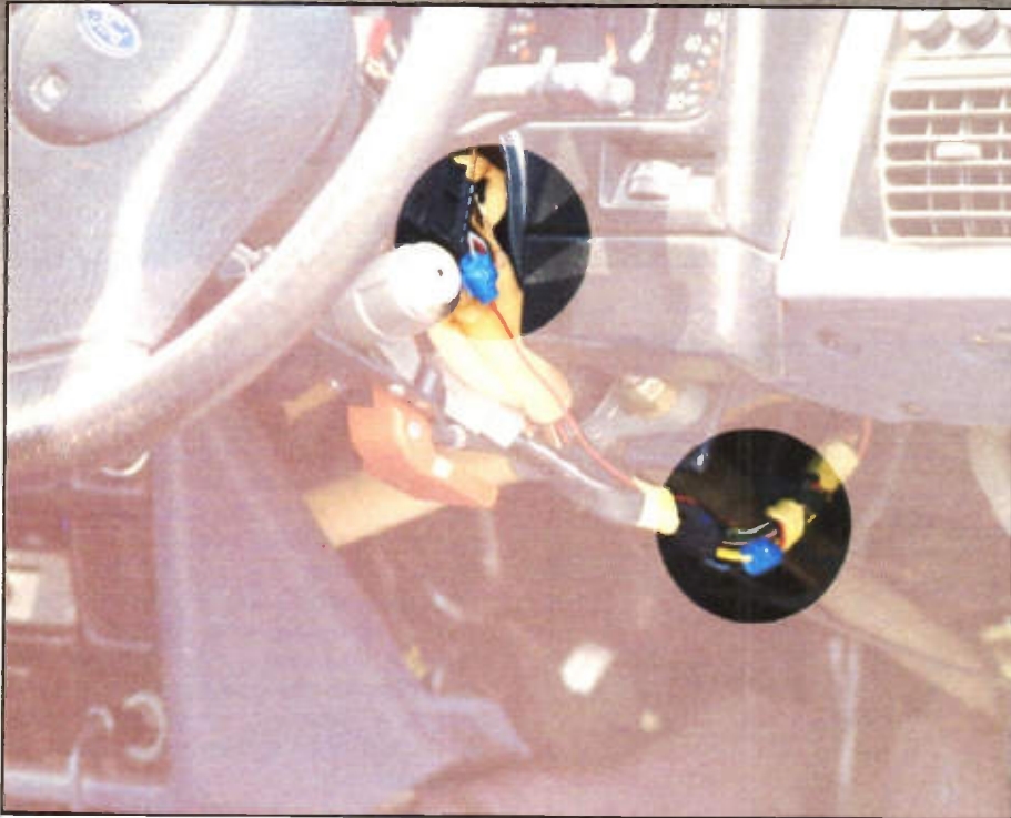
Photo 1. Connections to the sidelight circuit (left) and accessory circuit (right).
