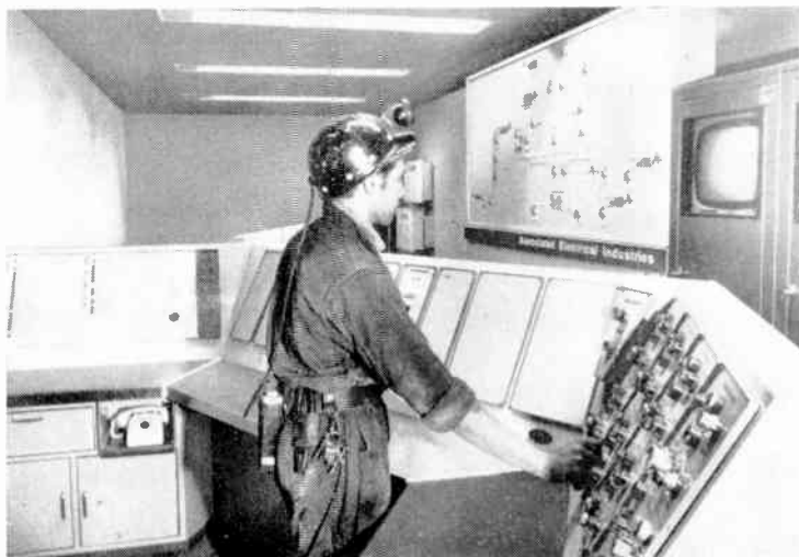
Fig. 2. The underground control room controls every main conveyor and the operating conditions of all underground equipment are displayed on the mimic diagram. The closed-circuit television screens on the right display the conditions at the pit-bottom bunker and those where the gate conveyors transfer the coal on to the trunk conveyor. Also located here is the base station for the two-way inductive-loop radio communication system, for maintaining contact with all the underground vehicles
