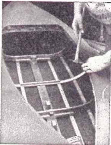
Fixing the deck canvas to the coaming frames around the edges of the cockpit
