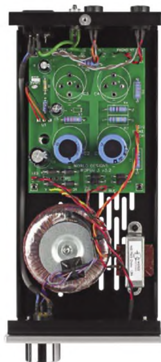
PSU3 with its toroidal transformer, smoothing choke (bottom right) and reservoir capacitors. No noise-producing voltage regulator chips.
