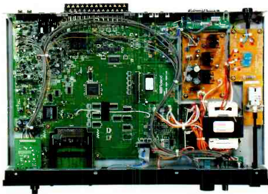
To the right are the AR-2000's PSU boards, to the left the large processing PCB stuffed with surface-mount ICs.
