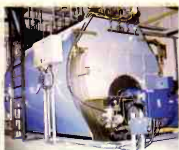
Just outside the press shop sits the high pressure steam boiler that feeds the 'stampers'.
