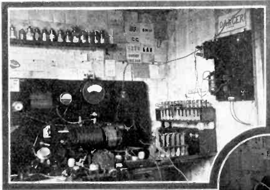
Fig. 4. A corner of the operating room. On the right can be seen the rectifying unit and the oil-filled condensers.
