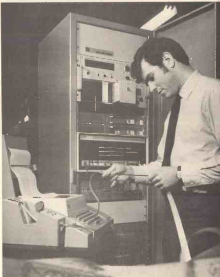
An engineer checks the paper tape output from a data logging system that operates in conjunction with a small computer. This particular type of installation can handle up to 1000 input signals, representing temperatures, pressures, flow rates, mechanical strain, liquid level, acceleration, etc. (Photo courtesy Solartron Electronic Group Limited)
