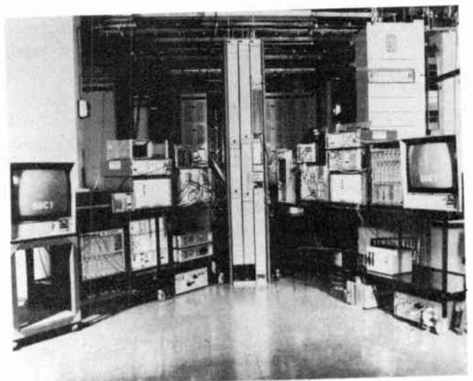
Fig. 5. The experimental equipment installed in Hitchin telephone exchange.
