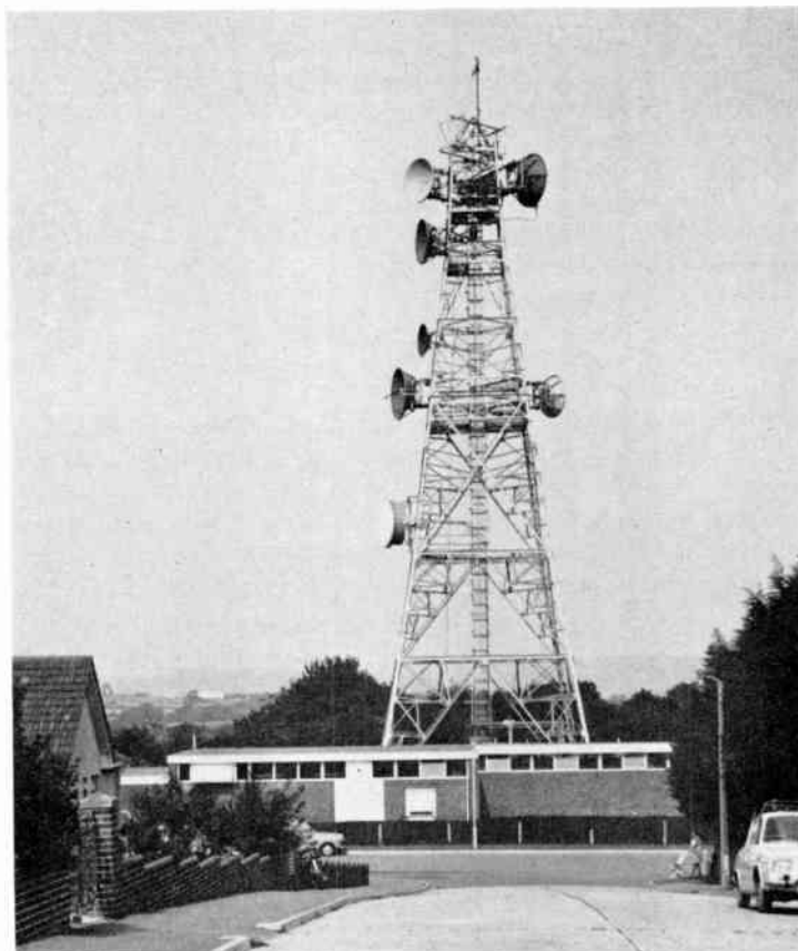
Fig. 1. Standard lattice steel microwave tower in the Post Office radio-relay network near Plymouth; the lowest dish antenna (1.5 m diameter) on the left-hand leg, with a protective radome, is installed for the new 11 GHz link to Caradon Hill.
