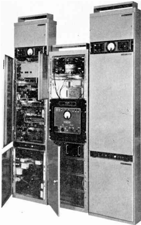
Fig. 8. General construction of trunk radio bays.
