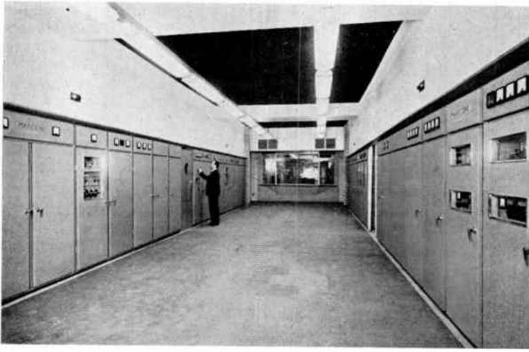
Fig. 3.—The Transmitter Hall at Crystal Palace; the Sound transmitters are on the left and the Vision transmitters on the right, with the Control Room in the background. The doors on each side lead to adjoining rooms from which the backs of the transmitters are accessible.
