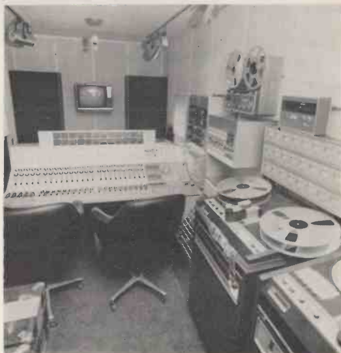
Equipment is, to say the least, comprehensive.
