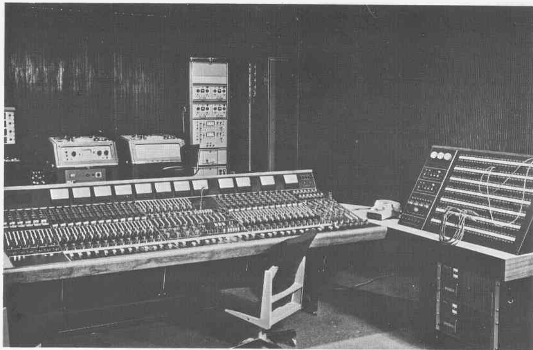
The new Rupert Neve console recently installed at Cine Tele Sound Studios, Bayswater, for music recordings, post sync and dubbing
