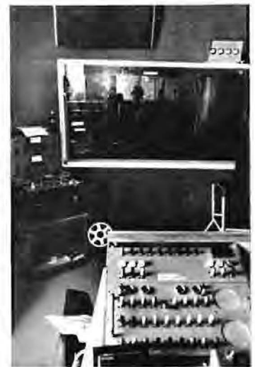
Interior of the Studio Republic control box
