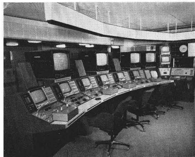
Fig. 3 Telecine control desk, showing six telecine control positions and one supervisory position
