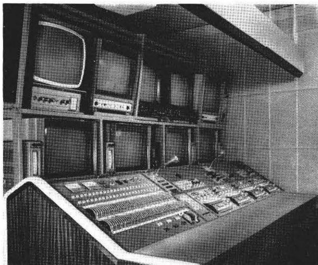
Fig. 6 Control console for lighting and camera positioning
