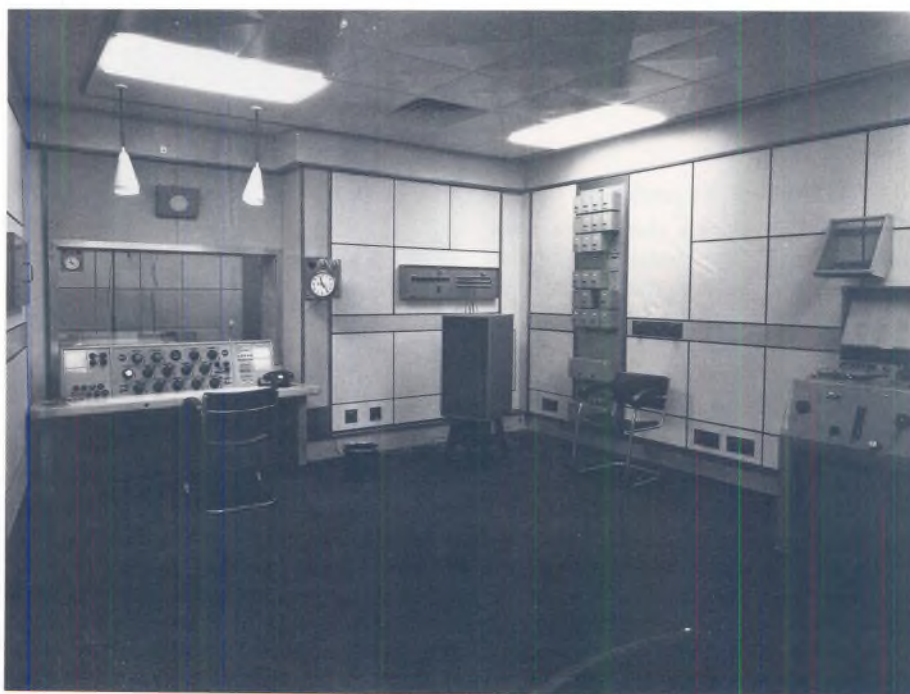
1963: The control cubicle of Studio B15 in BH Extension
