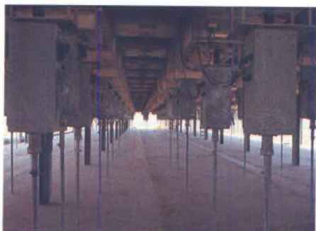
Cyprus: switch matrix looking between transmitter lines 203 and 211
