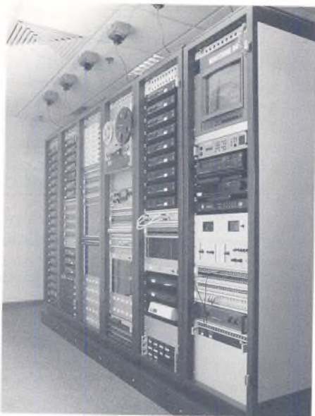
The headend equipment
