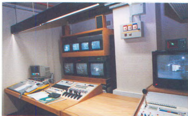
The completed Lighting & Vision control area
