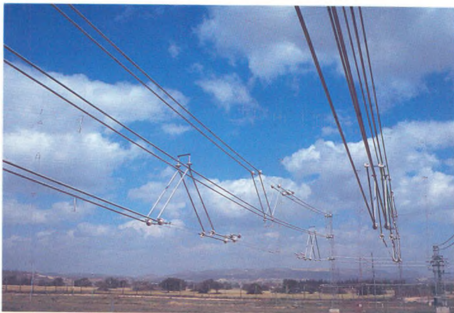
Cyprus: Array 54 6/7 MHz combiner at Zygi
