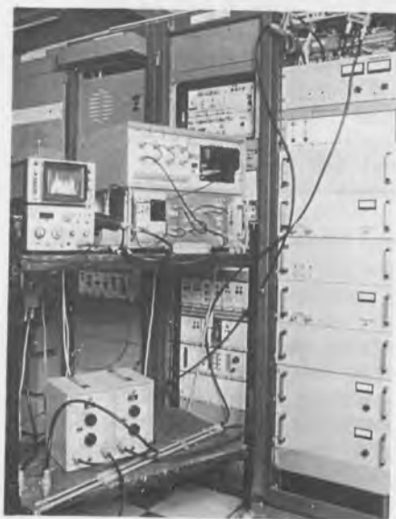
The additional transmission equipment installed at Wenvoe, for the two-channel sound with television experiment.
