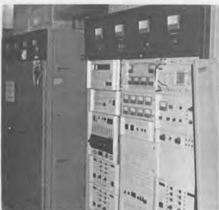
The new Marconi transmitter
