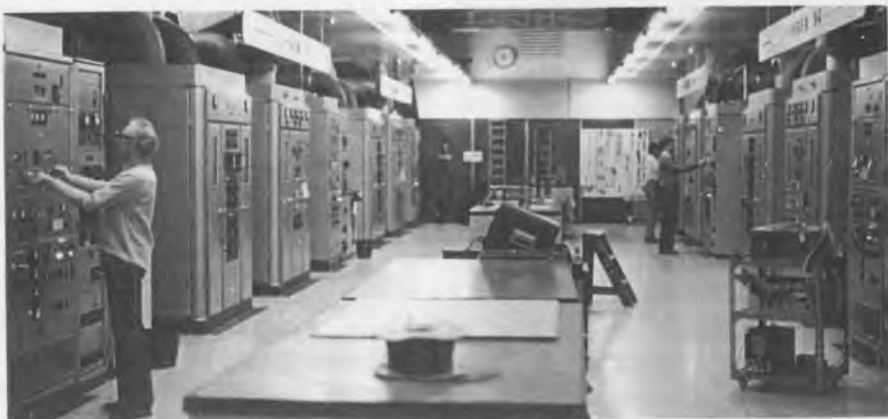
Engineers John Chantler, Jeff Chant and Phil Sandell adjust the 250 kW transmitters at Woofferton
