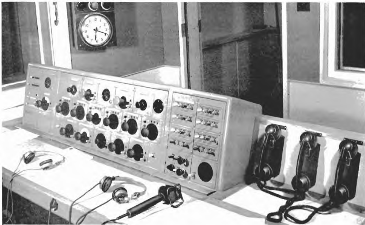
Plate 7.8. Control desk in Mixer Suite B.1., Broadcasting House
