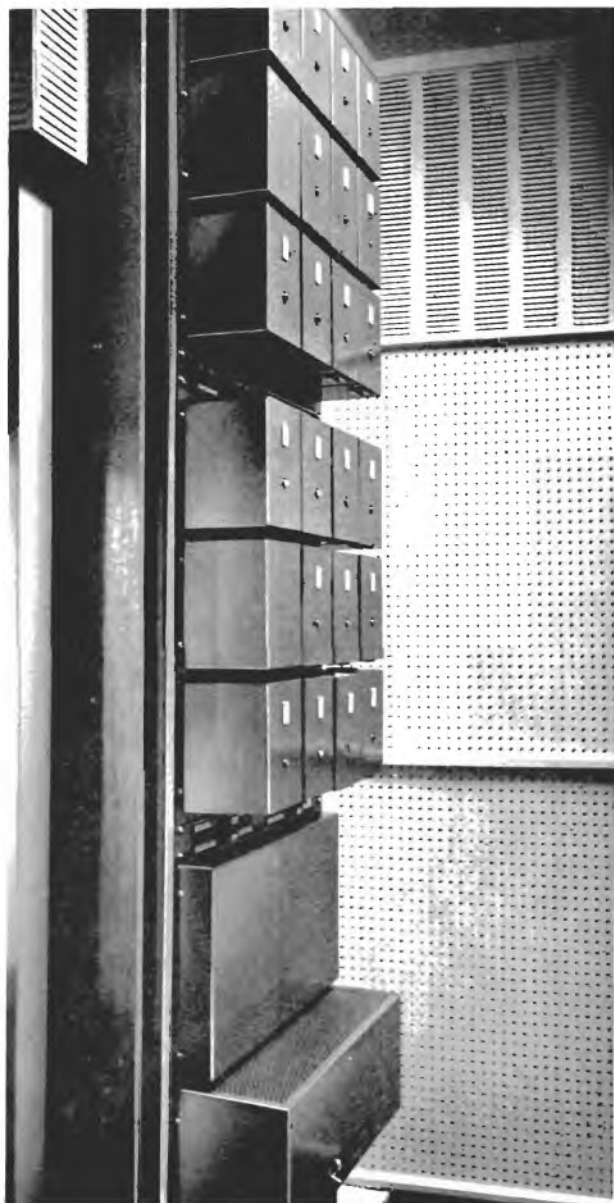
Plate 7.7. Type B equipment—amplifier rack, showing two groups of 10 amplifiers, standby amplifier and changeover switch, and mains unit
