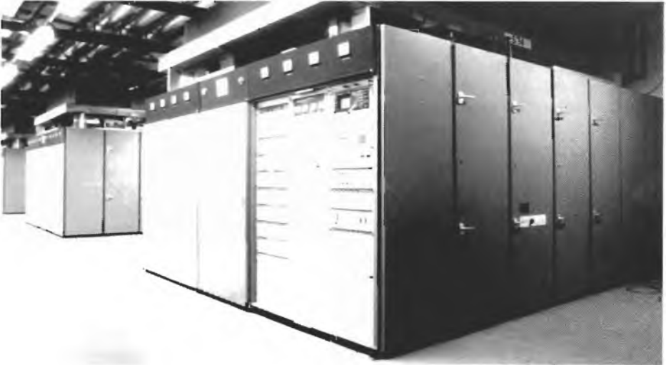
Three of the new remote controlled Senders installed in Skelton C. The sheer technicalities that enable these Senders to run unattended with all their functions controlled from London may be impressive to the engineers, but the visual impact is nil when compared to the giants of fifty years ago.
