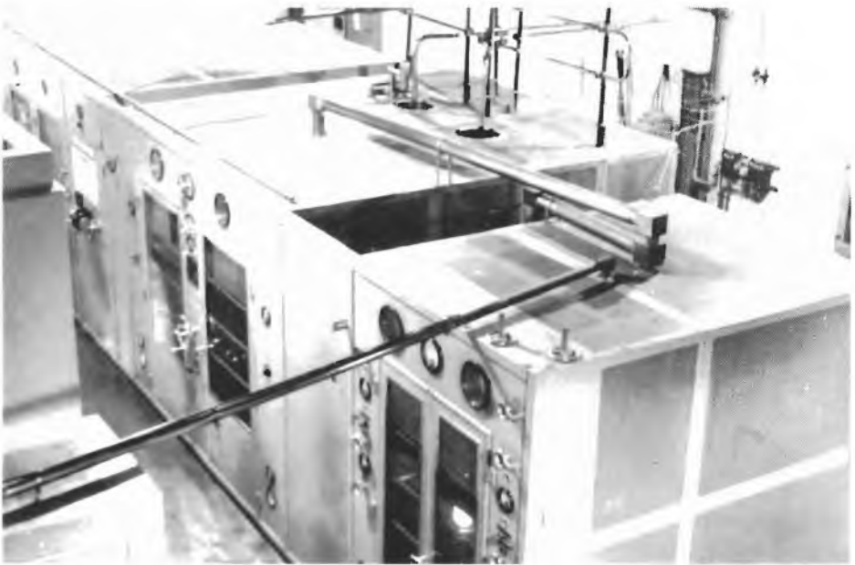
The coils shown in the photograph on page 12 were placed in the centre cabinet of the three shown in this overhead picture of Sender 65 at Skelton A (then OSE 8). The differences in the senders at Skelton A (when OSE 8) are easily seen when compared with a similar view of sender 75 at Skelton B (when OSE 9) on another page.
