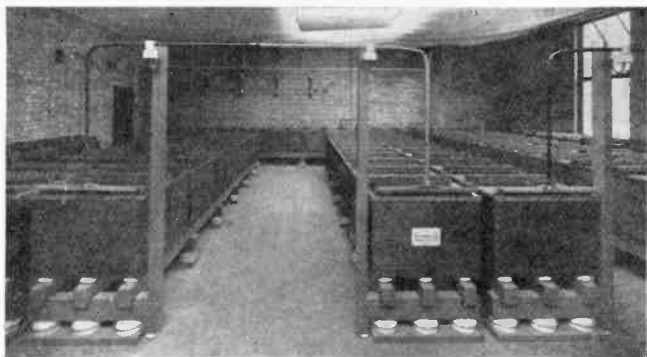
THE BATTERY ROOM AT BROOKMANS PARK
