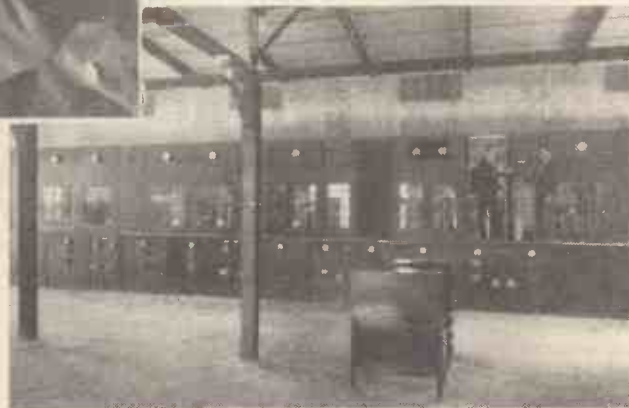
In the main transmitter hall of W8XO, the half-a-million-watt Cincinnati giant station now testing
