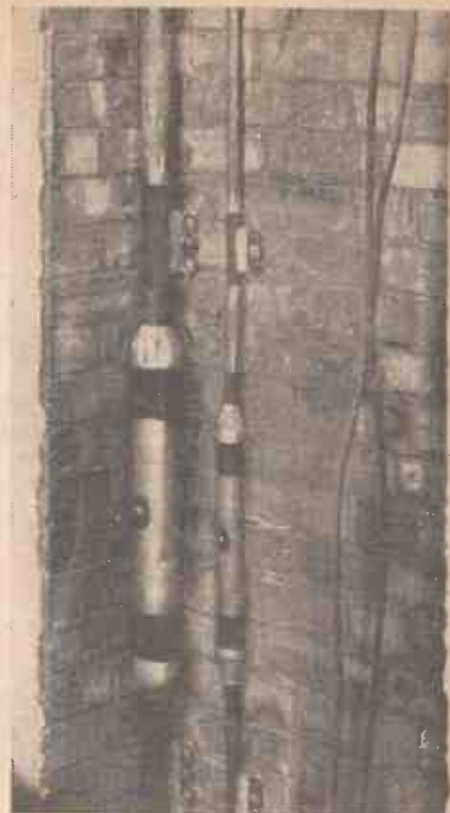
Here is an important link between Brookman's Park and the new Broadcasting House in Portland Place. Over 400 wires connecting the studios with the transmitter are covered by these conduits
