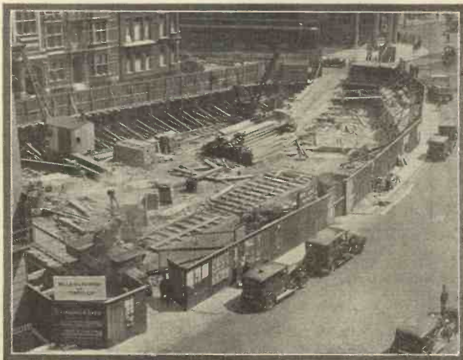
The new Broadcasting House—An actual start has been made of clearing the site for the new headquarters of the B.B.C.
