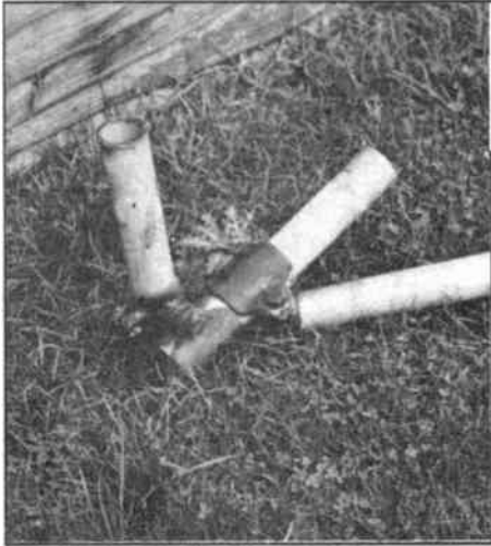
Photograph 6 The stand-off tube is attached to a further tube in the ground, with a swivel clamp forming a universal joint. This is shown after the mast had been lowered
