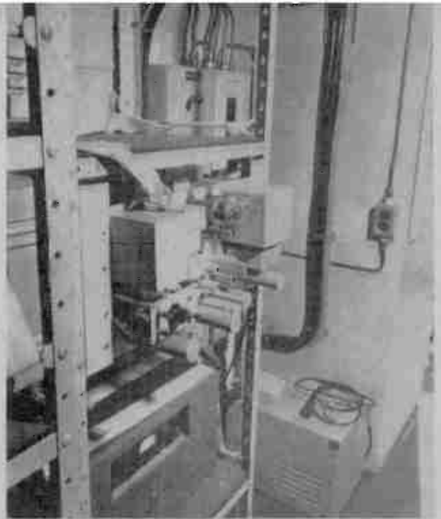
Rack 3 showing clamper and receiver power supply — power entrance in rear.
