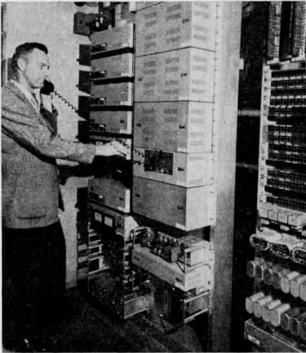
(Upper left): Russ MacDonald, Maritime Telephone and Telegraph Company's New Glasgow Central Office Foreman, uses service channel on the Collins' microwave equipment located at the Fraser's Mt. station.
