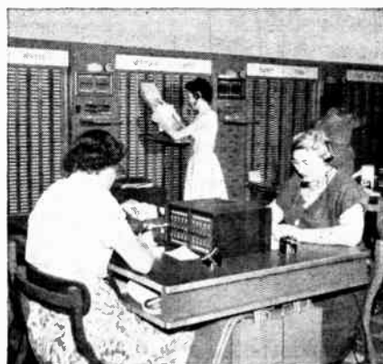
A new diol PBX system facilitates the handling of a greatly increased volume of calls. Shown here is part of the special customer contact service which required 24 positions of special answering equipment.
