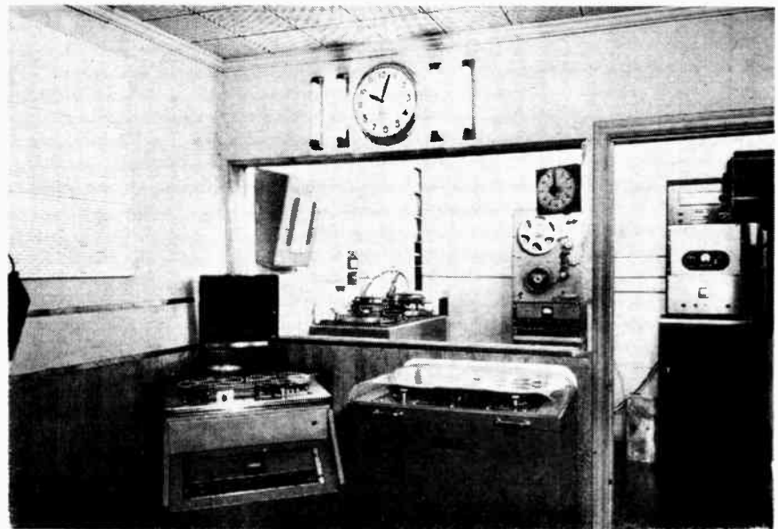
● Part of the wired music distribution studios of I.R.S. showing left two long-playing tape reproducers and in the rear tape duplicating equipment.
