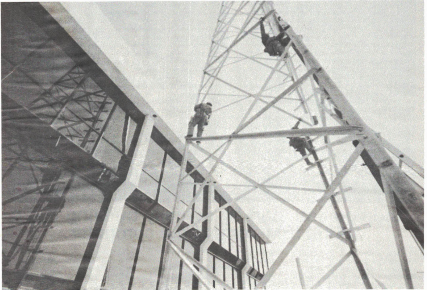
Installation of the cell site antenna at the Cantel head office in Montreal. This receives the digital signal from the mobile phone and relays it to the control centre.
