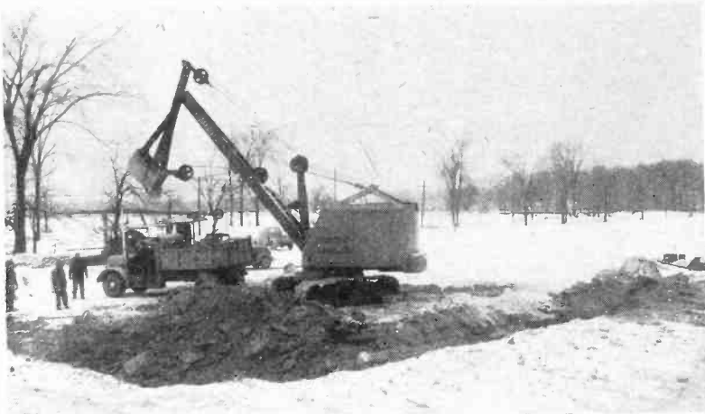
Here is the bull-dozer turning the first snow-laden sod for the new CFRB transmitter from where the Toronto station's signal will go out when the changeover to 50 Kilowatts on 1010 Kc. takes place this summer. The new transmitter, an RCA, type BTA 50-F, will be located at Clarkson, 20 miles west of Toronto just off the Lake Shore Highway.
