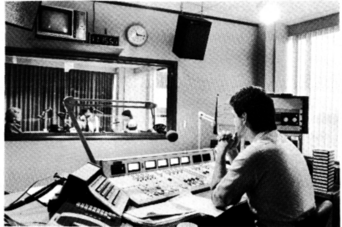
Production control room is equipped with an Auditratics 110A production board, Otari 5050 MK III 4-track tape machine, Otari 5050B-II 2-track and full track, ITC cart machines, Technics SP-15 turntables and EV Sentry 100 monitors.
