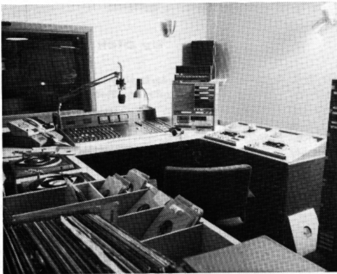
Master Control Room
