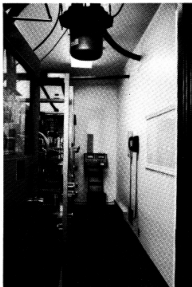
Main transmitter building.
